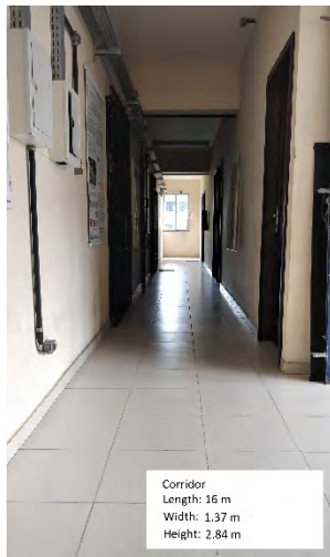
FIGURE 2. Environment For The First, Second And Fifth Measurement Campaigns (In The Corridor).
