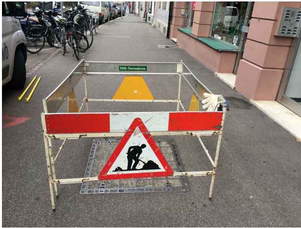
FIGURE 15. Closed service shaft cover made of steel and concrete.
