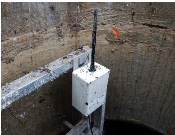
FIGURE 19. Uninviting conditions: Synchronous LoRa mesh sensor node mounted at a manhole ladder in a sewer shaft (temporary installation).
