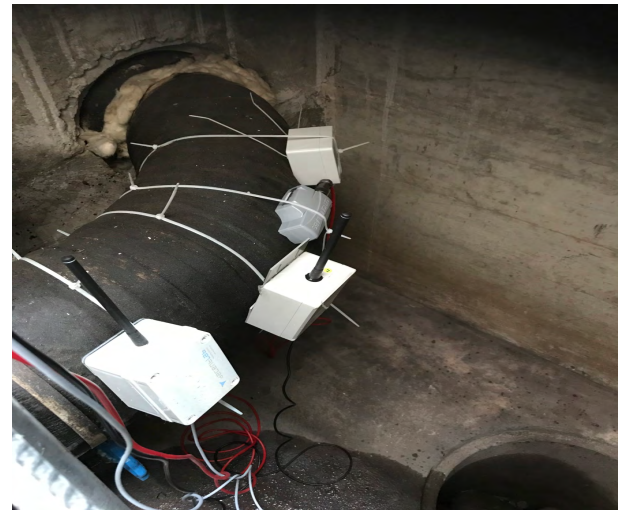
FIGURE 14. Synchronous LoRa mesh and LoRaWAN reference nodes in the service shaft in 3 m depth were mounted next to each other.
