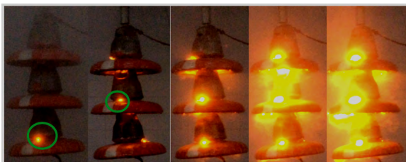
FIGURE 9. The flashover process of RTV insulator string with five percent fan-shaped damage.
