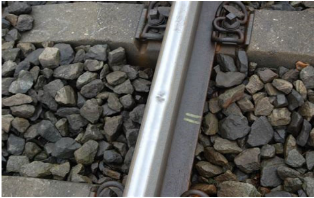
FIGURE 1. Defects on rail surfaces.
