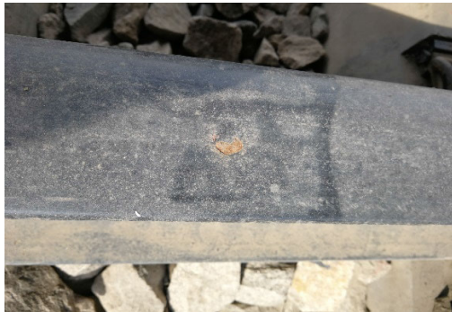
FIGURE 27. Defects at a distance of approximately 60 m.
