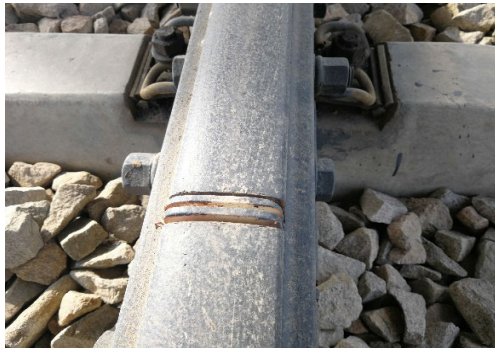
FIGURE 26. Defects at a distance of approximately 20 m.
