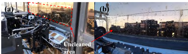
FIGURE 20. (a) Uncleaned area of glass panel, and (b) closed view.
