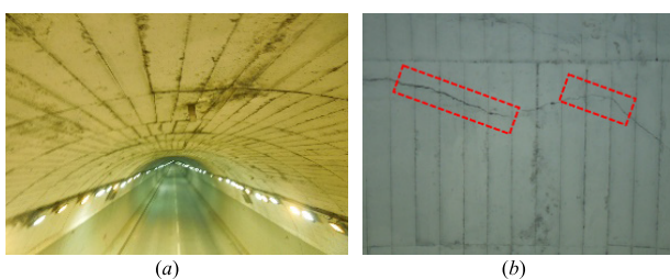
FIGURE 2. Tunnel concrete structure. (a) The tunnel passage. (b) The tunnel concrete surface with seams and cracks.
