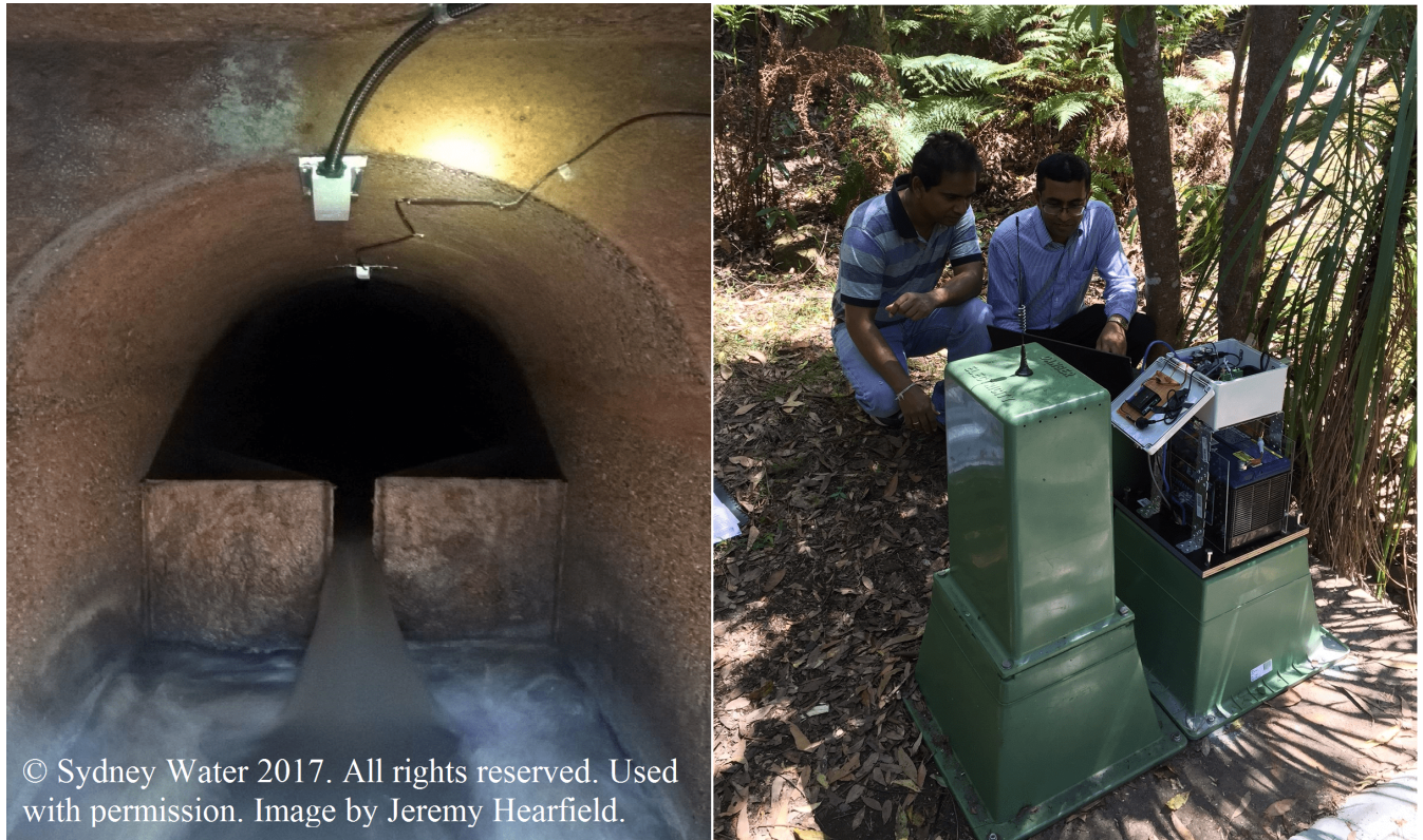
FIGURE 1. Field deployment of sensor suite displaying the sensing system installed inside the sewer pipe near the head-space and access station constructed outside the sewer pipe for data monitoring and acquisition.
