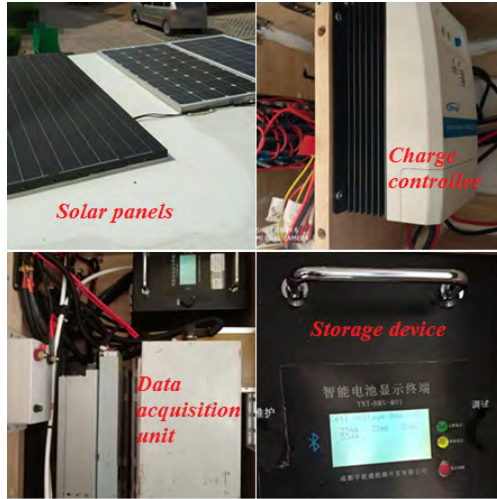
FIGURE 4. Our data collection and testing platform (located at 35.28N, 113.95E, 75mASL, capacity with 480Wp).
