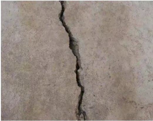
FIGURE 7. The original image of the crack.
