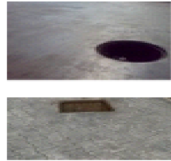
FIGURE 8. Inputs of manholes.
