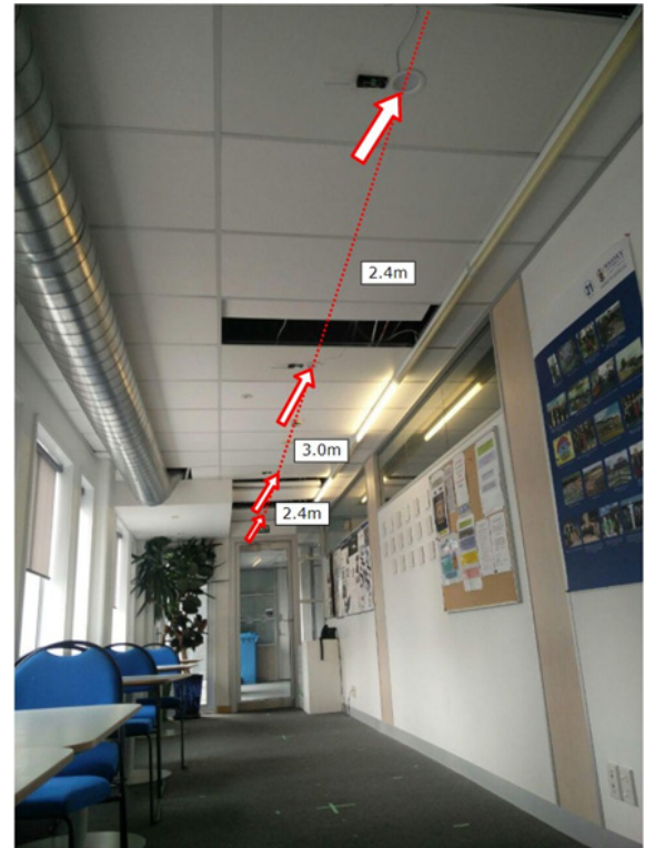
FIGURE 2. Anchor nodes installed in hall.
