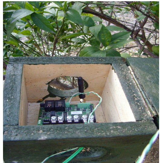
FIGURE 5. Air temperature and humidity sensors deployment.
