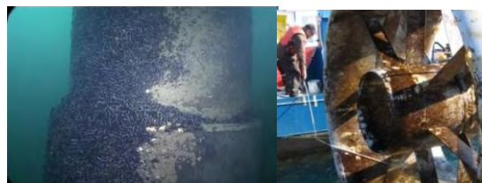
FIGURE 7. Biofouling & Erosion for MCECS [39].
