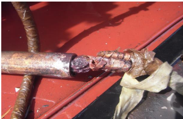
FIGURE 7. A-phase lead connector of the transformer on the high-voltage side.
