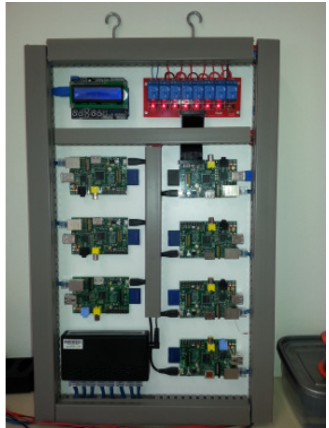
FIGURE 5. Complete NPi-Cluster, assembled on a wall-mount frame (version with Raspberry Pi 1 nodes).
