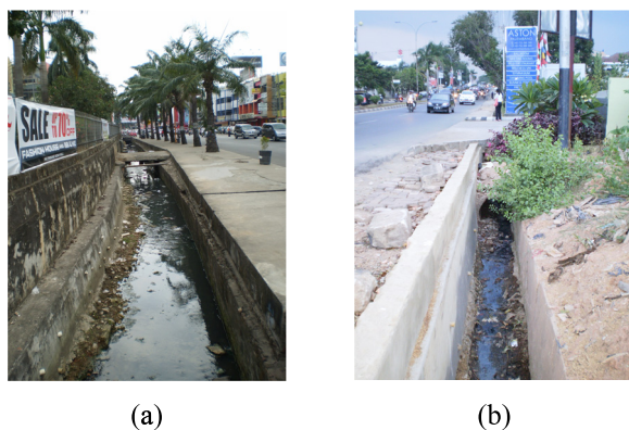
FIGURE 1. Pictures showing two examples of open-trench drain that can be widely seen in Asian cities. (a) A wider drain. (b) A narrower drain.
