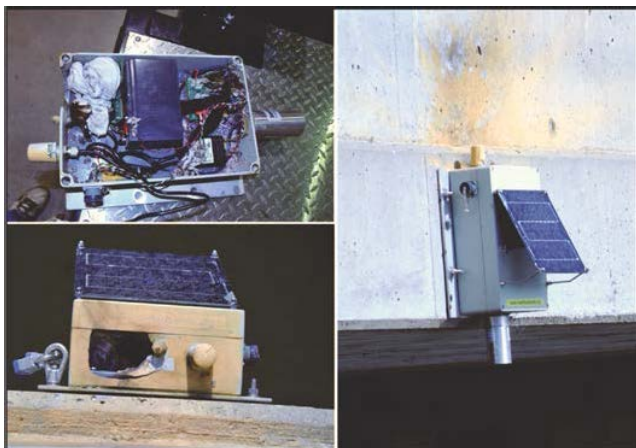
FIGURE 26. Fig. 26. Photographs of a BMRSS unit damaged by vandals.
