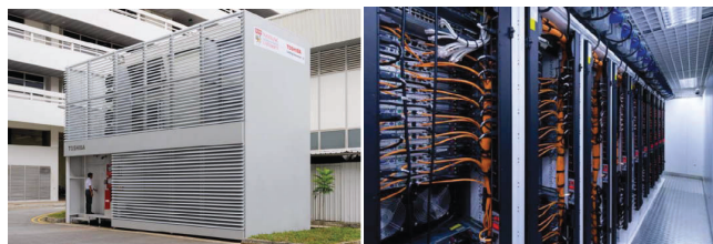
FIGURE 1. A modular data center was built at Nanyang Technological University (NTU) for system/testbed research. The testbed hosts 270 servers organized into 10 racks.
