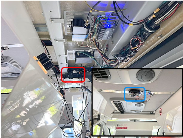
FIGURE 6. Installation in a NAVYA autonomous minibus. Hardware setup consists of a NVIDIA Jetson AGX Xavier device (highlighted in the red box) and a D-Link DCS-4625 fisheye camera (highlighted in blue box).
