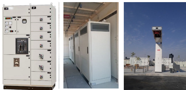
FIGURE 13. Charging infrastructure deployed in qatar.
