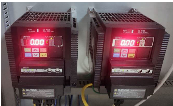
FIGURE 5. Omron 0.75 kW frequency inverters in the control unit.
