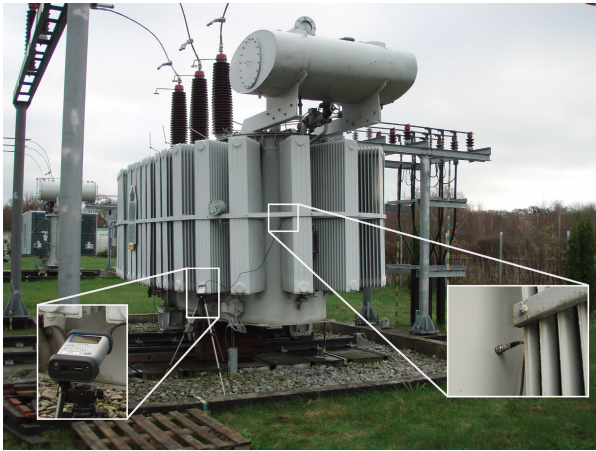
FIGURE 1. Transformer TR-16000/110, 115/16.5 kV, 16 MVA with accelerometer sensor and recorder.
