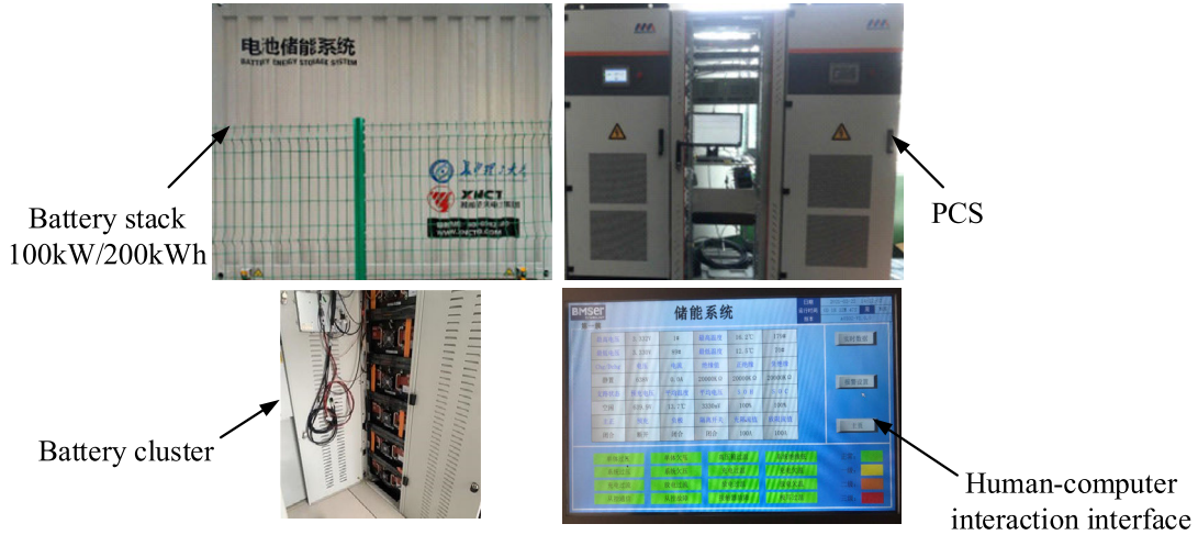
FIGURE 21. Energy storage system platform and interface of measurement system.
