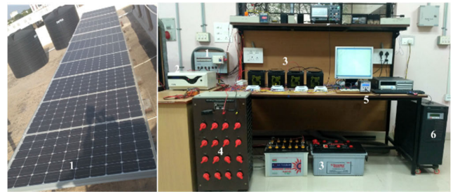
1. PV Array, 2. MPPT Charge Controller, 3. Batters, 4. DC load, 5. Data Logger, 6. Grid connected Inverter
