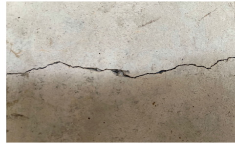
FIGURE 19. Crack on concrete bridge column present under the bridge deck.
