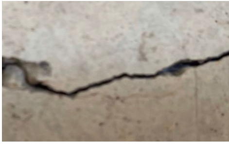
FIGURE 20. Cropped crack portion belongs to crack shown in Fig. 19; The cropped image includes almost similar crack characteristics from the training sample.
