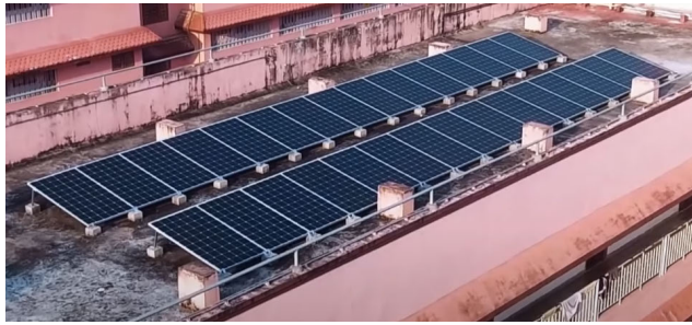
(a) Rooftop solar panel in Hostel block
