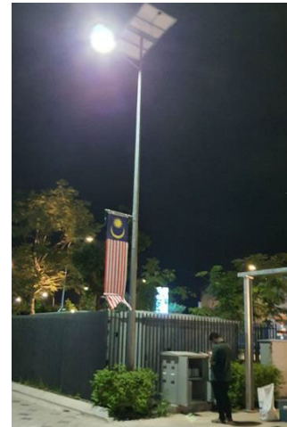
FIGURE 15. System installed onSite.
