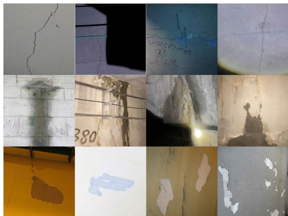
FIGURE 8. Example of tunnel surface defect images.
