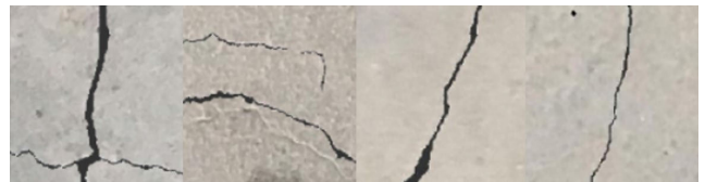
(b) Synthesized cracks
