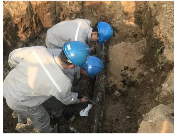
FIGURE 2. Site photo of buried gas pipeline leakage experiment for theory verification and validation.
