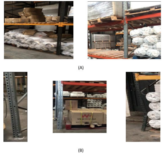
FIGURE 2. Racking data sample internal class inspection (A) normal (B) damaged racking.
