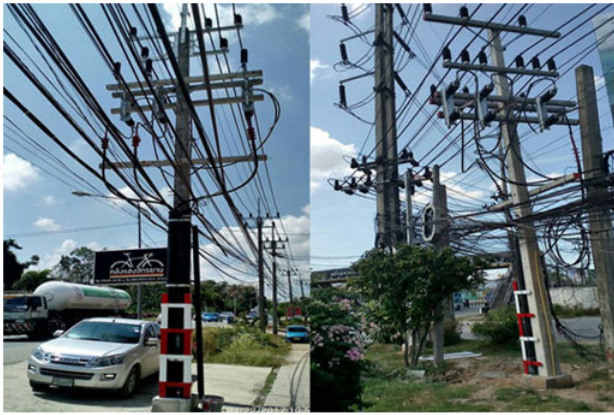
FIGURE 1. The multi-feeder structure of the distribution lines (author’s personal picture).
