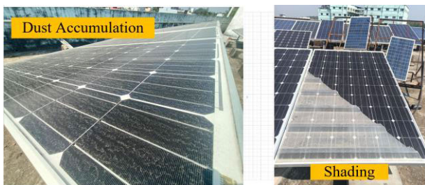
FIGURE 32. Fault creation on PV panels.
