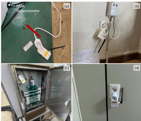
FIGURE 2. Examples of low-cost IoT seismometer (LCIS) installation locations: (a) building floor, (b) wall outlet, (c) utility pole, (d) temporary wall.
