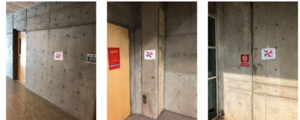
FIGURE 5. Images with labels to indicate elements are scanned by the GPR device.
