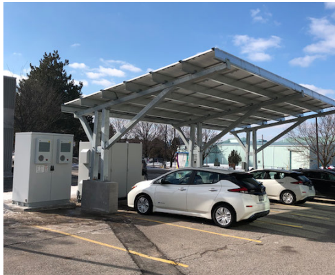
FIGURE 8. Photo of commercial building with BESS (left), solar (top), and Nissan Leaf with bi-directional charger (right).
