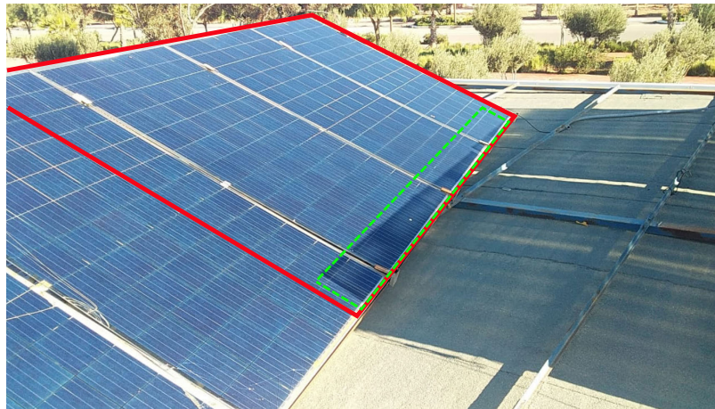
FIGURE 11. Shading of the photovoltaic string at Green Energy Park’s test bench.
