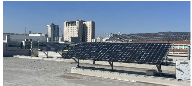
FIGURE 6. PV power system with 1.99 kW Mono-S.
