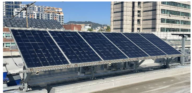
FIGURE 7. PV power system with 1.77 kW Bi-S.
