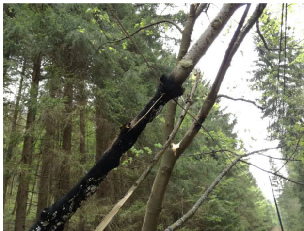
Fig. 1. Fallen tree on medium voltage overhead line with covered conductors.
