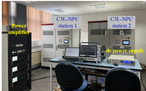
Fig. 17. Three-terminal MVdc configuration, including two C3L-NPC converter stations and a dc power supply operated at current-controlled mode.
