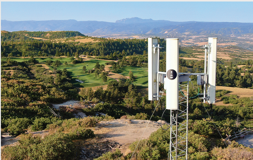
Dish Network Corp., owner of this 5G cellular tower, is in a high-stakes skirmish with Elon Musk's SpaceX over the use of the 12-gigahertz spectrum band.
