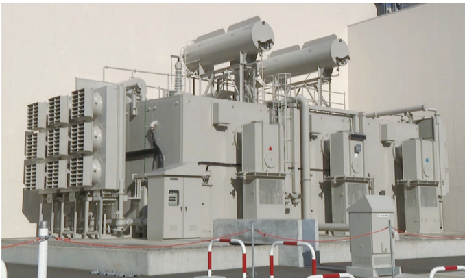
Figure 3. Converter transformer at the Hida CS.
