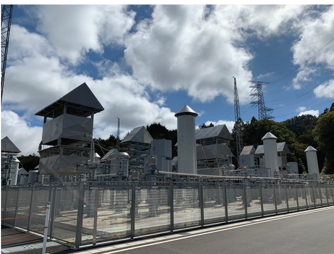
Figure 5. AC filters with covers and triangular roofs for protection against possible snow damage.
