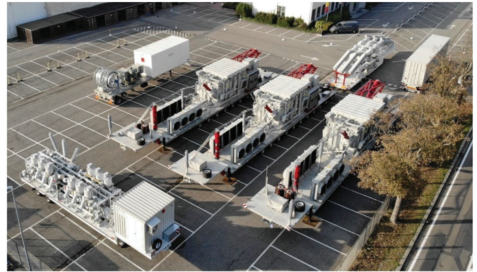
Figure 2. CG Belgium designed and built a 400-kV mobile substation on seven trailers (with permission of CG Holdings Belgium NV).
