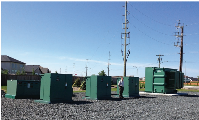
Figure 3. 115-kV and 69-kV, 10-MVA HVPT and 138-kV and 72-kV, 12.5-MVA PODS manufactured by PTI Transformers LP (Regina, Canada) for utilities in central Canada.
