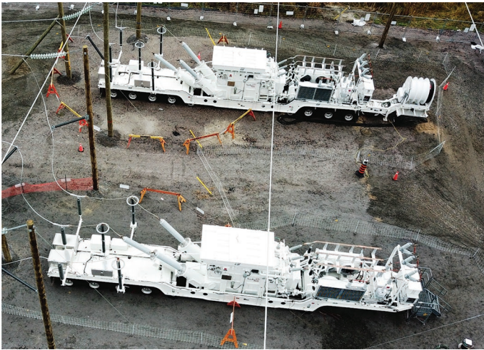
Figure 1. Hydro One Networks Inc. deployed two 230 × 115 kV, 30-MVA mobile transformers designed and built by PTI Transformers LP (Winnipeg, Canada) in an emergency situation at Minden substation, Toronto area, in August 2018. Published with permission of Hydro One Network Inc.
