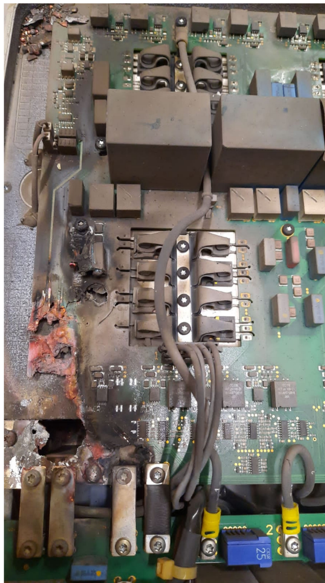
Fig. 10. Destroyed inverter SMA.
