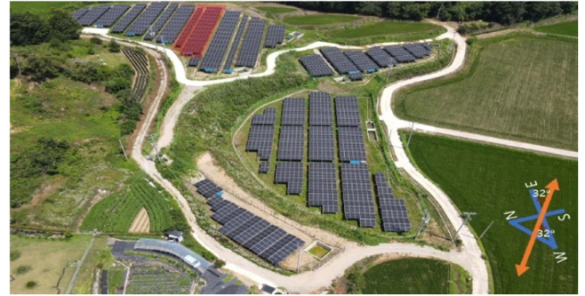
Fig. 10. Large-scale PV power plant installed at azimuth the angles of 122^\circ and 302^\circ .
