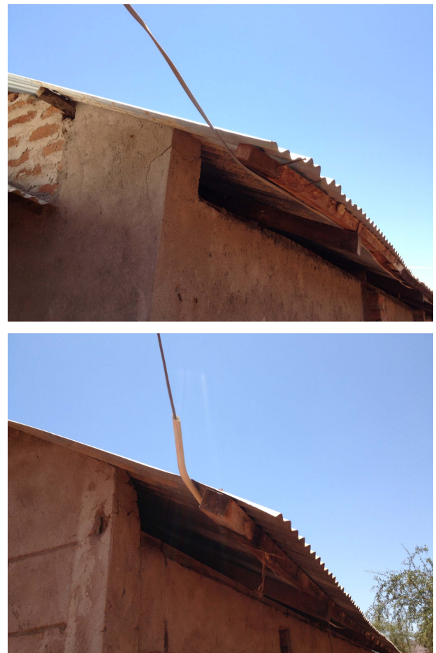
Fig. 5. Top: example of poor local contractor quality and poor understanding of electrical risk. Bottom: typical field remediation of poor-quality contractor deployment.
