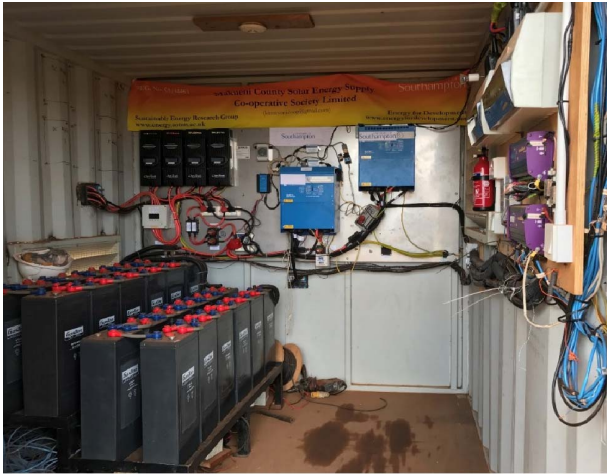
Fig. 3. Kitonyoni plant room comprising four charge controllers, 48-V battery bank, and twin inverters. Data monitoring system is on the right-hand side below consumer units of twin distribution circuits. Diesel generator is located on the other side of central bulkhead added to the container.
