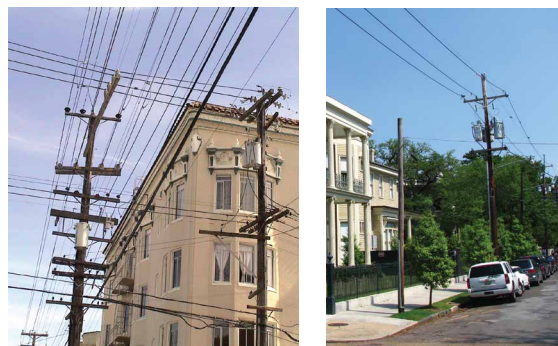
Fig. 2. Urban distribution grids in San Francisco (left) and New Orleans (right), where the same wood pole usually holds both MV and LV feeders.
