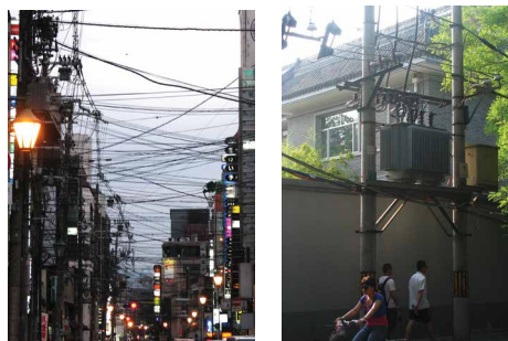
Fig. 1. Urban distribution grids in Tokyo (left) and Beijing (right), where both MV and LV grids, transformers, and switchgear are frequently aerial.
