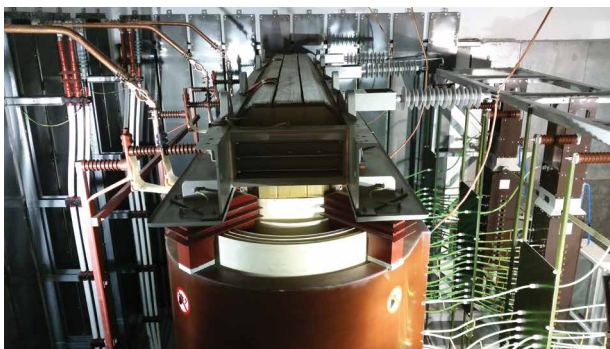
Fig. 22. Top view of a 72.5-kV, 34-MVA dry transformer located in downtown Seville. The separate on-load tap changer using vacuum switches is located on the right while the steel sheets intended to mitigate the magnetic field can be seen vertically arranged on the walls.
