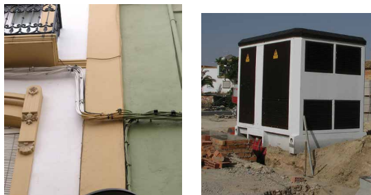
Fig. 3. Facade-mounted, LV aerial bundled cables (left) typically found in towns and medium-sized cities of some European countries, and underground MV cables (right) entering a compact, prefabricated concrete-made secondary substation, customarily used in urban and suburban areas in Europe.
