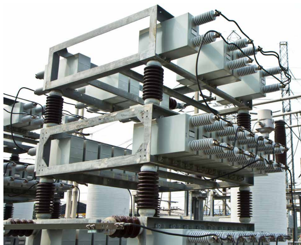
Fig. 1. A capacitor bank of an electric power transmission substation. Digital image courtesy of 123rf.com.
