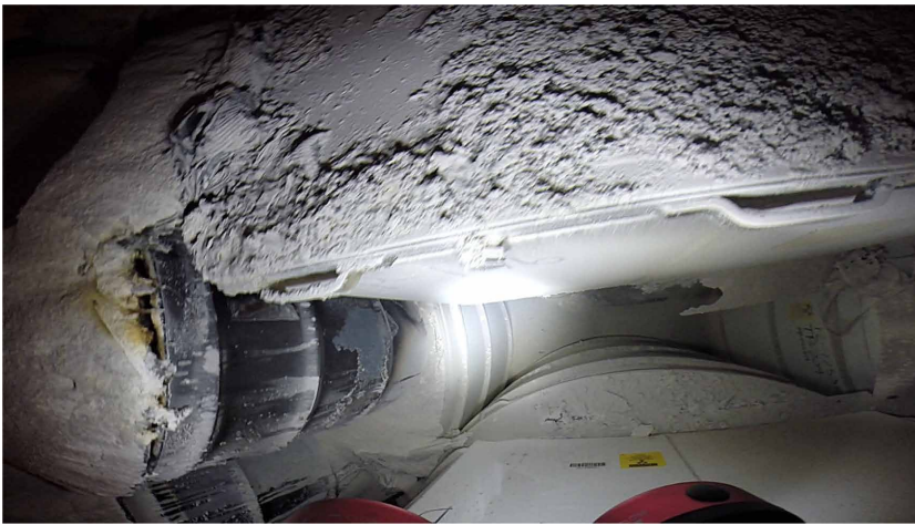
Photograph of a waste container at the Waste Isolation Pilot Plant, USA, with its lid unsealed and apparent heat discoloration taken by the U.S. Department of Energy on May 15, 2015. Source: http://www.wipp.energy.gov/wipprecovery/photo_video.html
