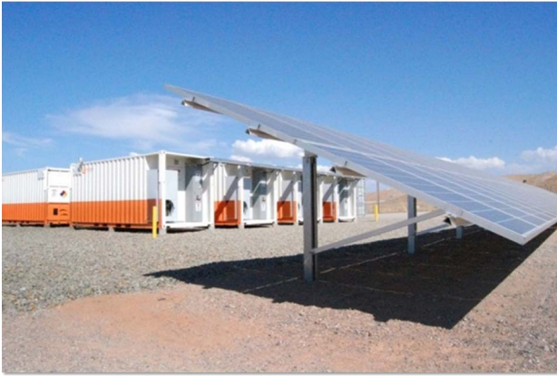
Fig. 4. Public Service New Mexico PV and energy storage site, Albuquerque, NM, USA.
